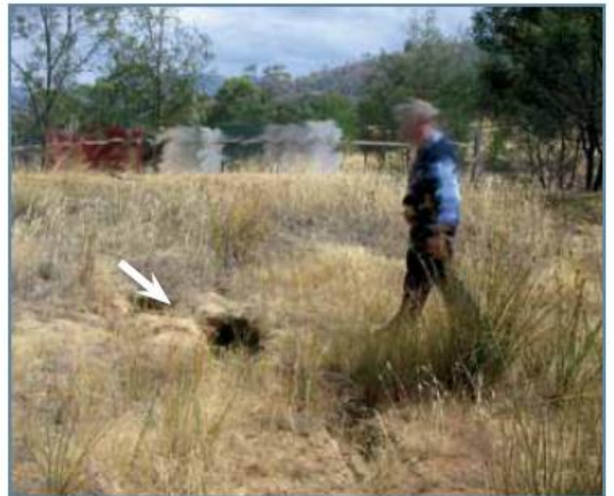
Figure 33. Typical small dam failure. Note piping through the side wall of the dam. This dam was constructed using dispersive clays derived from Triassic sandstone.
