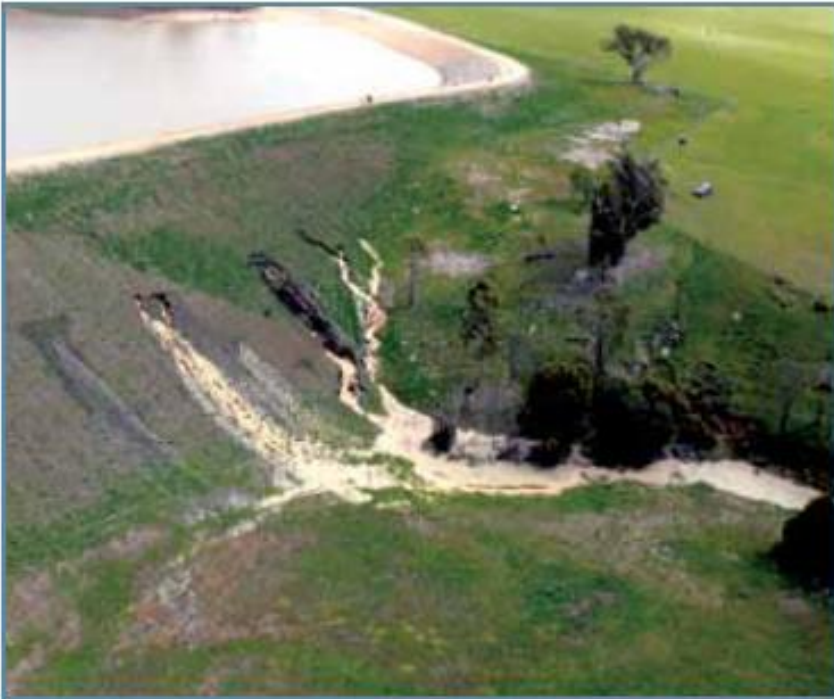
Figure 35. Failure of Blackman Creek dam (source: Davies Brothers). In 2005 the Blackman creek dam failed, resulting in the evacuation of Tunbridge. Doyle and Cumming (unpublished 2005) indicate the cause of the failure to be variability in the compaction of a slightly to a moderately dispersive soil layer, combined with rapid filling of the dam with low electrolyte water.
