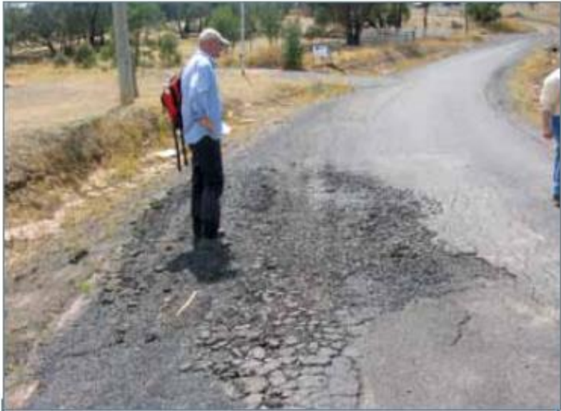
Figure 25. Road surface breaking up due to construction on dispersive clays. This section of road is repaired 2-3 times a year.
