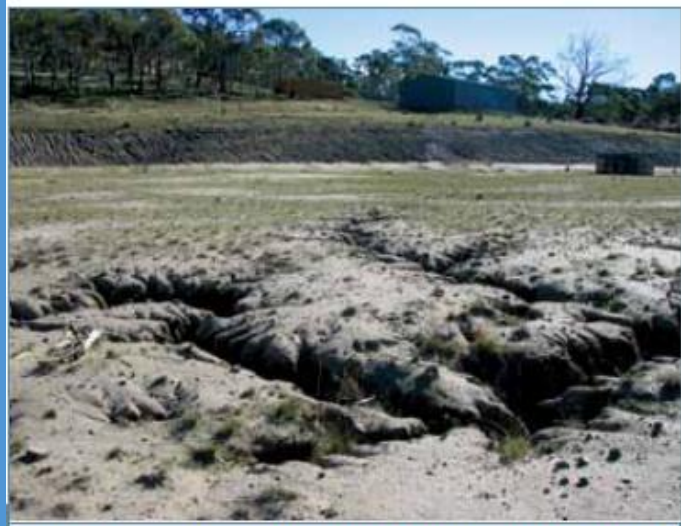
Figure 18. (Same site as Figure 17) Tunnel erosion in footings intended for a large building. Erosion resulted from ponding of rainwater on highly dispersive fill. The fill contains a number of narrow slots (up to 1.2 meters deep) caused by surface water 'dissolving' through the footing.
